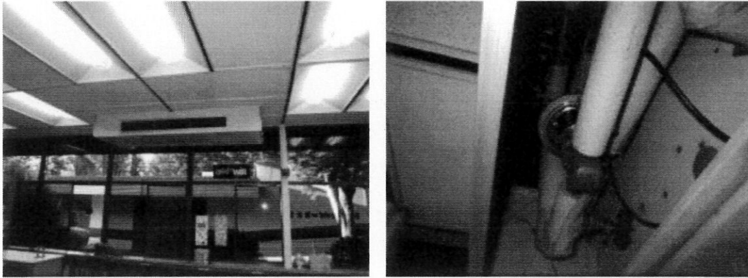
Figure 2.1: Typical Unit Ventilator Fan Coil (L) and Hydronic Valve (R) Used in Classrooms
